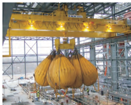
Overhead Bridge Cranes
